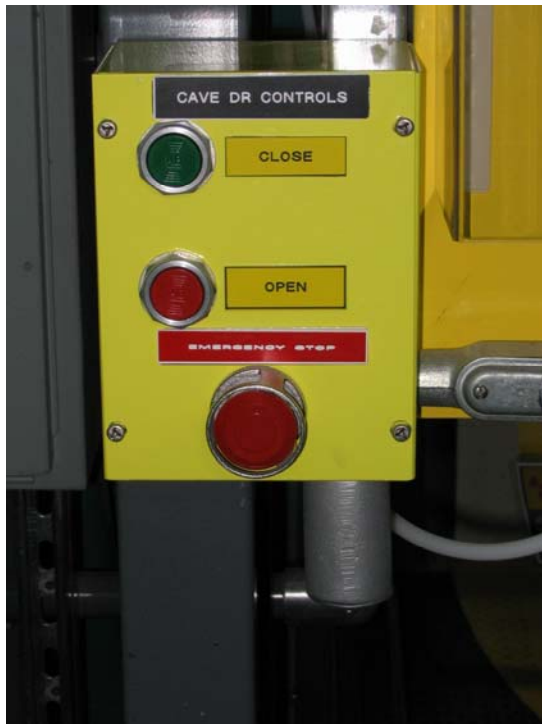
Cave Door Control Station
