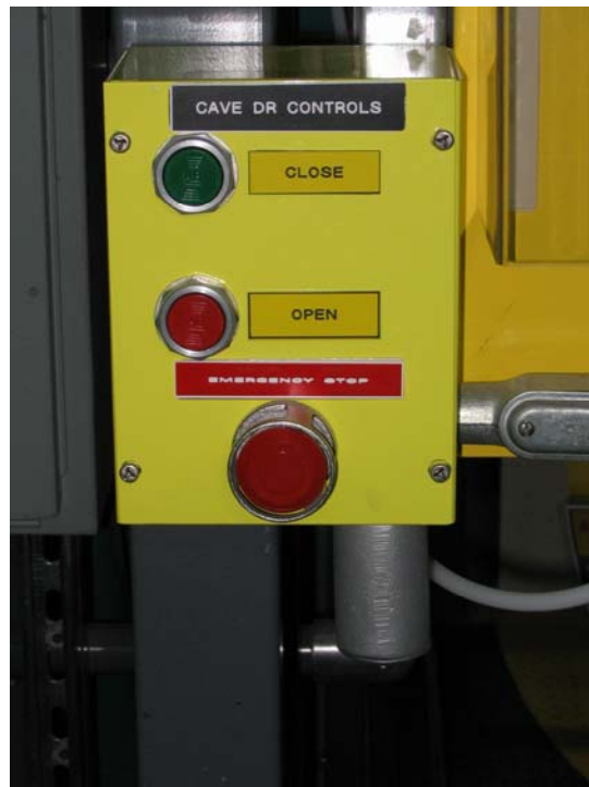
Cave Door Control Station
