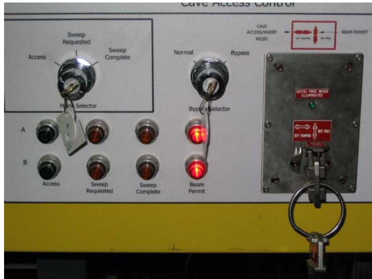
Beam Permit status lights illuminated
