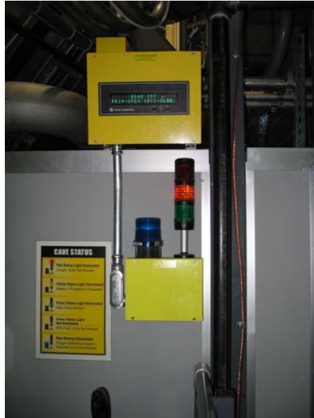
The exterior stack light, the blue Oxygen Deficiency Hazard strobe light and the PPS message board.
