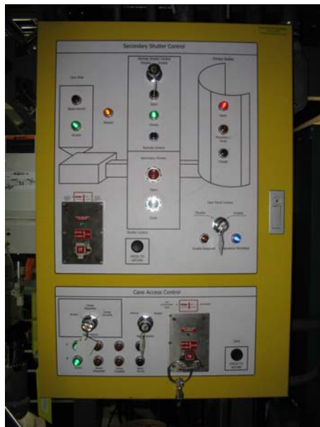
The Instrument Personnel Protection System User panel, which is used to open and close the secondary shutter.
