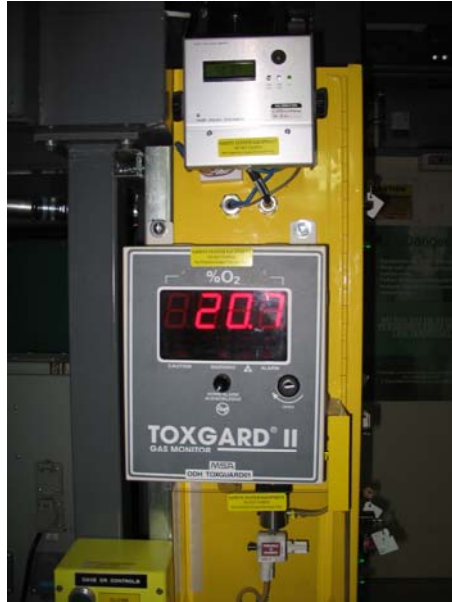
The O2 level monitor and the Radiation level monitor, which display conditions within the instrument cave.
